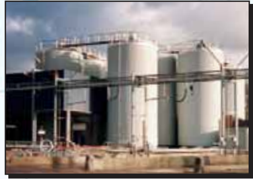
Level measurement on storage tanks
